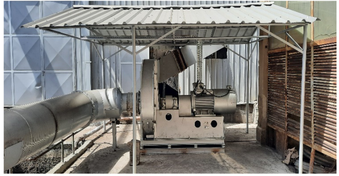
Picture 6: Electrical fan
