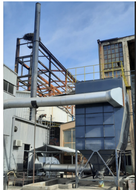
Picture 2: Stack AA2 to Boiler
