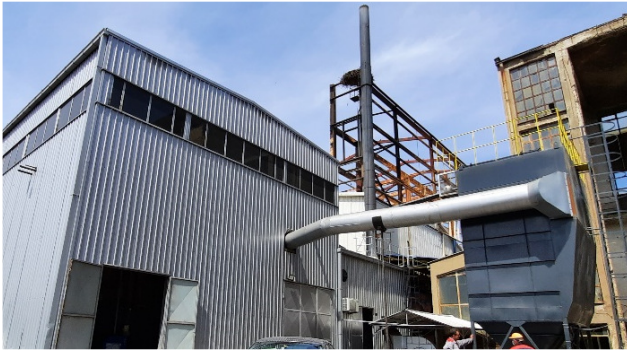
Picture 5: Flue gases abatement equipment (bag filter)
